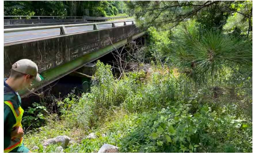
PATH team member descends beneath I-85 Access Road in order to field verify the feasibility of the proposed alignment.
