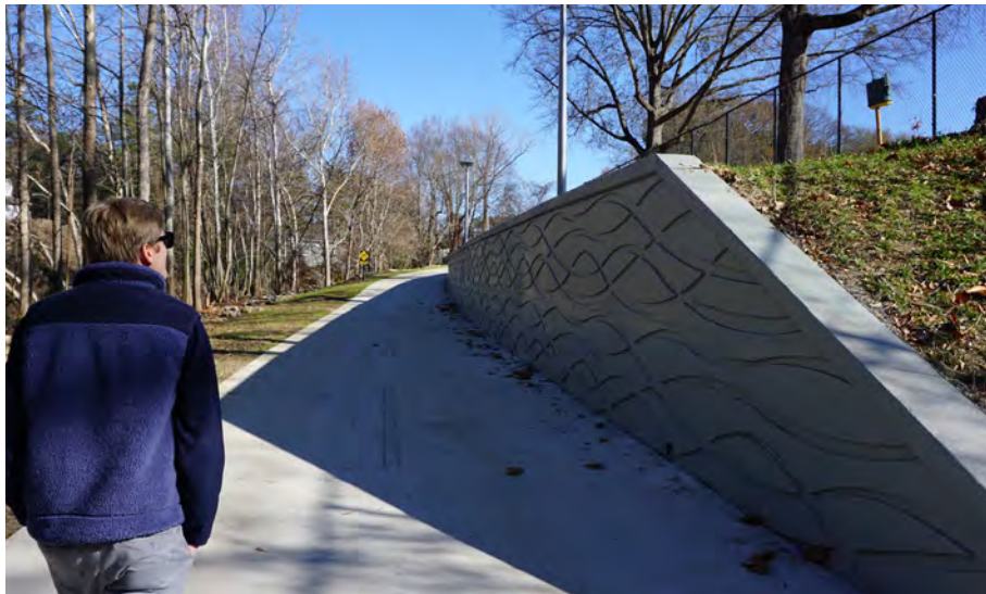
Example of Aloha Pattern wall finish along the PCG in Brookhaven, GA
