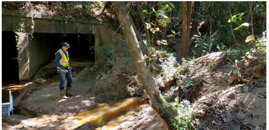
The PATH team conducted field work both around and through the box culvert under Spaghetti Junction
