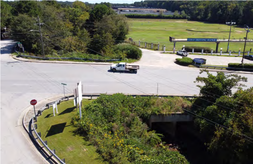
Existing conditions of a double box culvert under Northcrest Road, facing east. The proposed trail will utilize the south (right) box to cross, similar to the proposed conditions under Pleasantdale Road.
