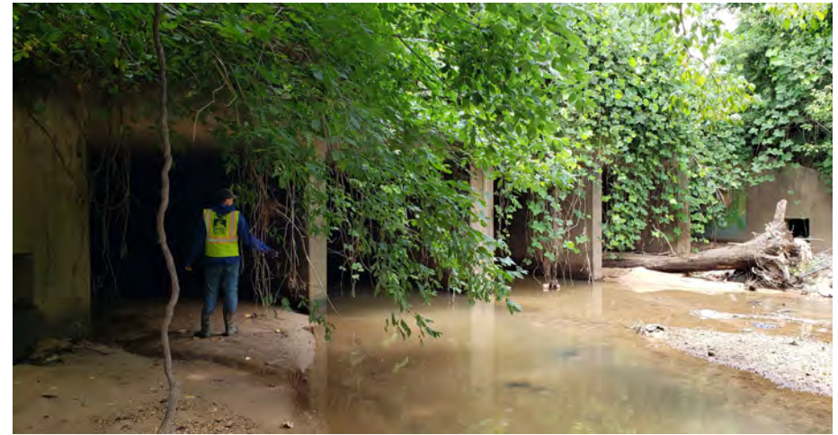
Existing five box-culvert under Chamblee Tucker Road, facing north-west. A flood study is advised to confirm that the eastern most box may be reconfigured for a 10'-0' wide multi-use trail.
