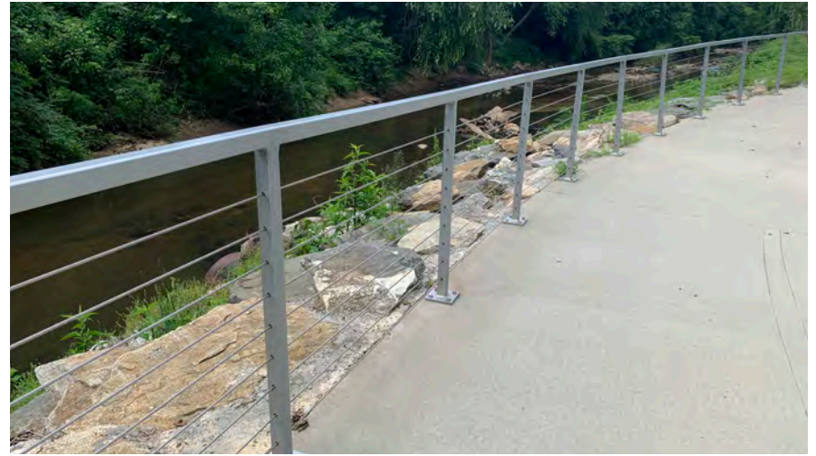
Shop painted metal post and cable handrail used along the PCG in Brookhaven, GA
